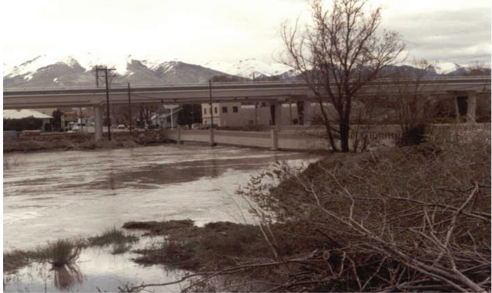
Figure 11.3.12 Flood Conditions: Note Pier Settlement.
