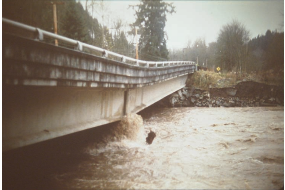
Figure 11.3.14 Movement of a Substructure Unit
