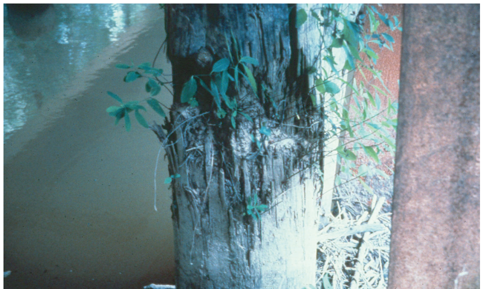
Figure 11.3.27 Deteriorated Timber Piling
