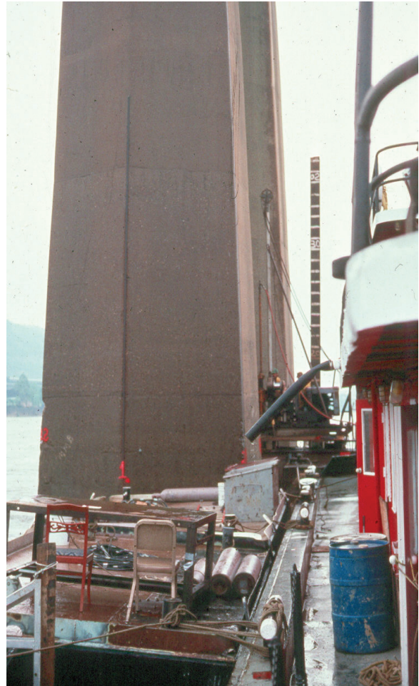
Figure 11.3.10 Permanent Reference Point (Bolt Anchored in Nose of the Pier, Painted Orange)
