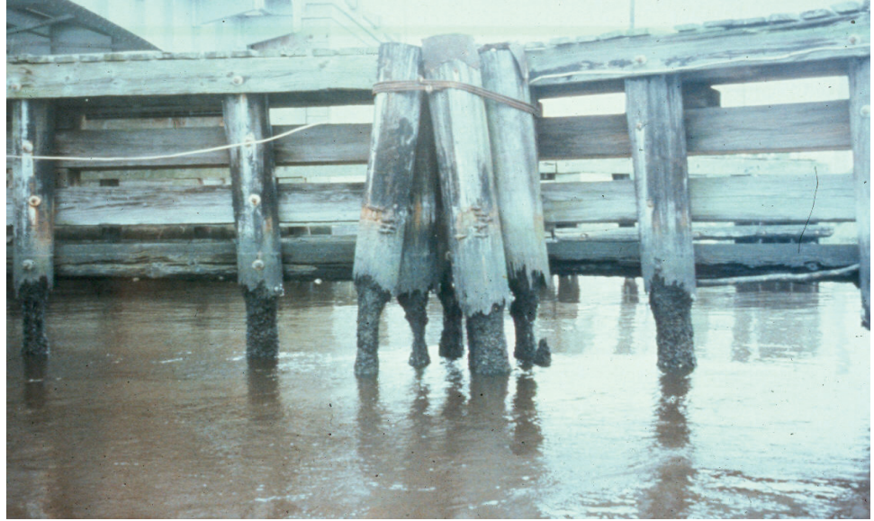
Figure 11.3.23 Damaged Protective System
